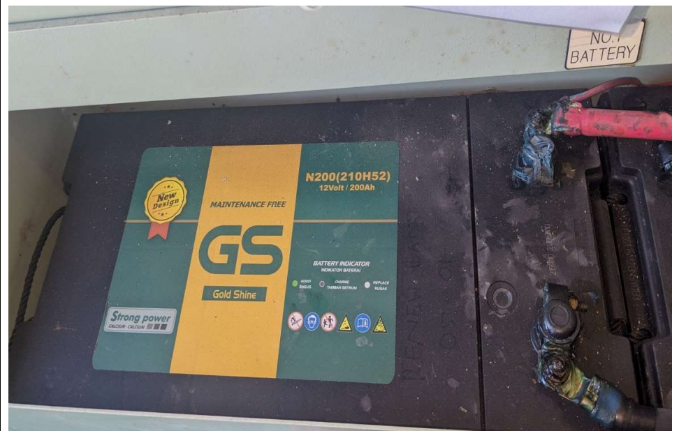
Battery Em'cy Generator
