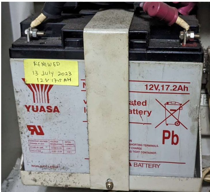
Backup Battery Alpa Lub Main Engine
